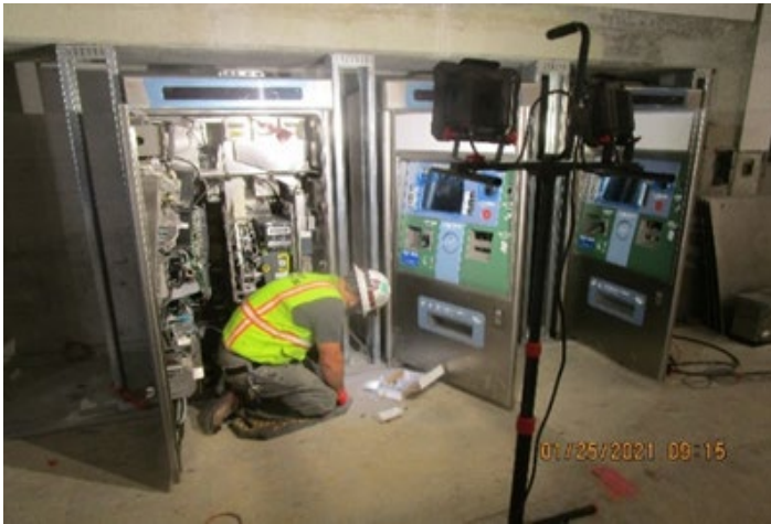
MLK STATION – Anchoring and installing ticket vending machines at the Free Area.
