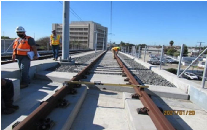
La Brea Station - Field site walk with WSCC QC & Metro CM team at La Brea OP SB track STA 202+00 checking track conditions on guideway (looking south).
