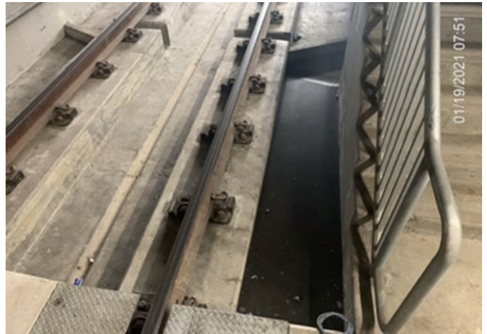
UG4 – Stagnant water condition at south portal NB track.
