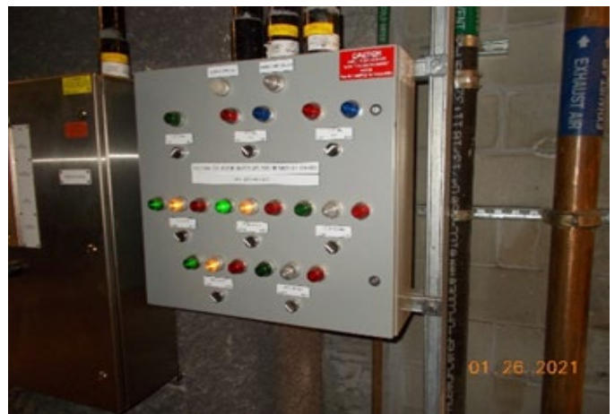
Vernon Station – Troubleshooting limit switches.
