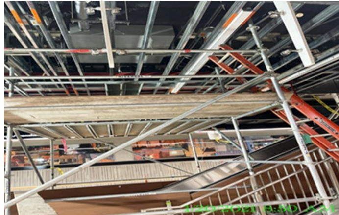
EXPO STATION – Continue LED light fixture installation at the platform ceiling grid.
