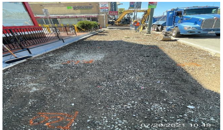
MLK STATION SITE – Fine grading and preparing for concrete placement at the southeast corner of Crenshaw Blvd and Martin Luther King Blvd.
