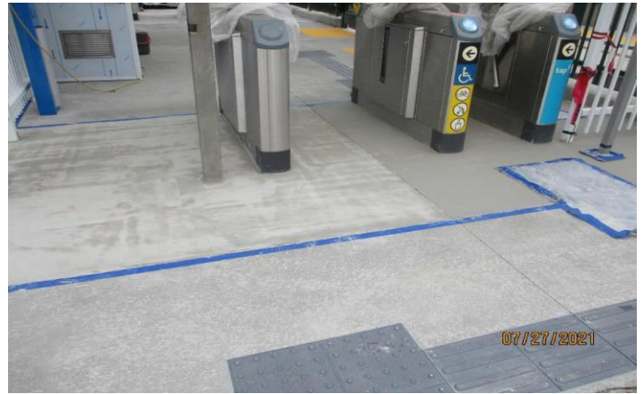
LA BREA STATION – Concrete finish work at the La Brea Station west TVM kiosk.
