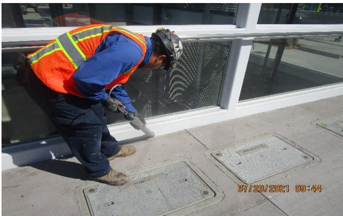
LEIMERT PARK STATION – Caulking and sealing isolation joints along the perimeter of Elevators 1&2 at the plaza.
