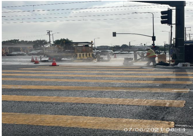
PARK MESA – Continue applying thermoplastic striping to the westbound pedestrian crosswalk on Crenshaw Blvd and Slauson Ave.
