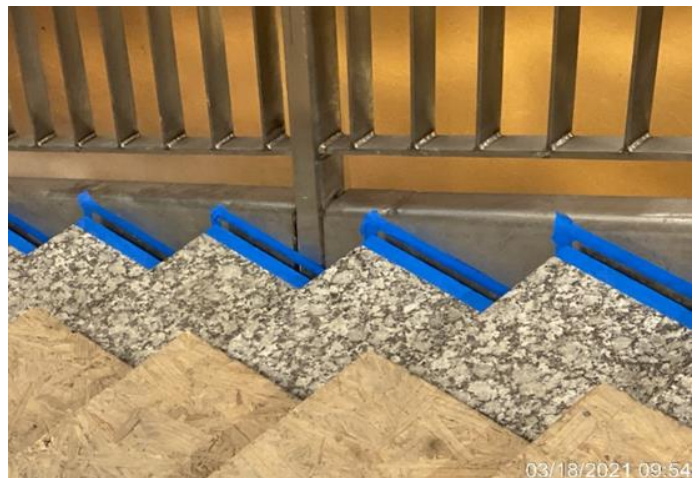
EXPO STATION – Caulking the tread joints of Staircase 3 from concourse to platform.
