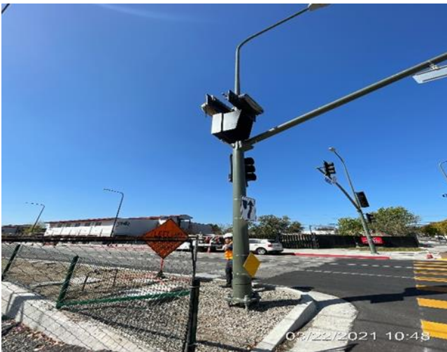
PARK MESA – Installed train warning signal overhead at the intersection of Crenshaw Blvd and 57th St.
