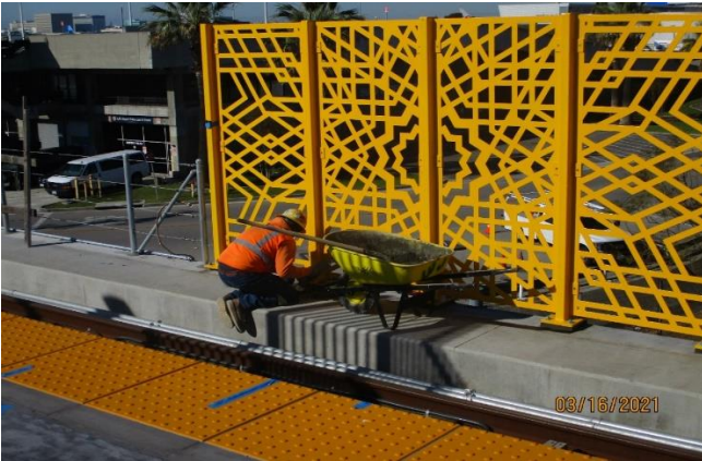
AVIATION STATION – Grout packing the fence post bottoms for the decorative fencing at the Aviation Station platform. Facing west.
