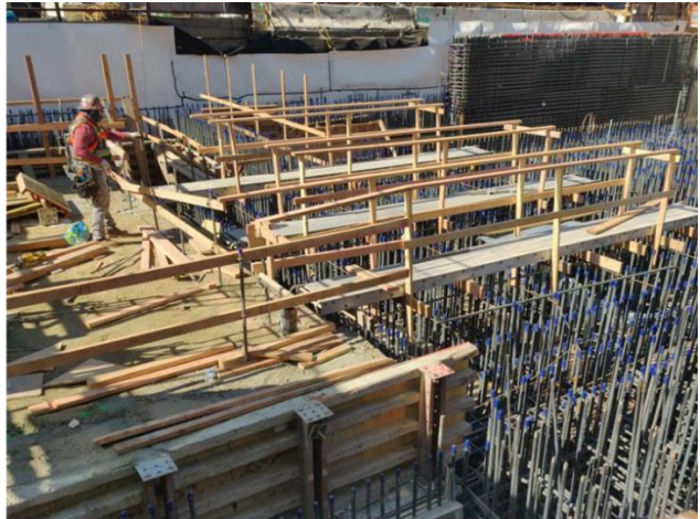
Access platforms over Load Transfer System (LTS) at Historic Broadway Station
