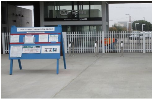
AVIATION STATION – Tightening fencing bolts at the Aviation Station Plaza. Facing east.
