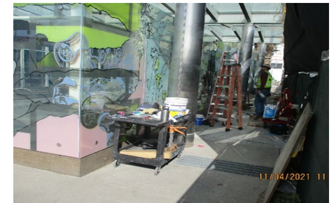
MLK STATION – Caulking and sealing the art glass panels around the perimeter of the main entrance plaza canopy
