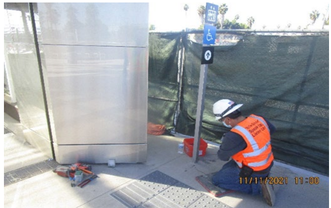
EXPO STATION – Grounding ADA pole sign adjacent to the main entrance door at the plaza.
