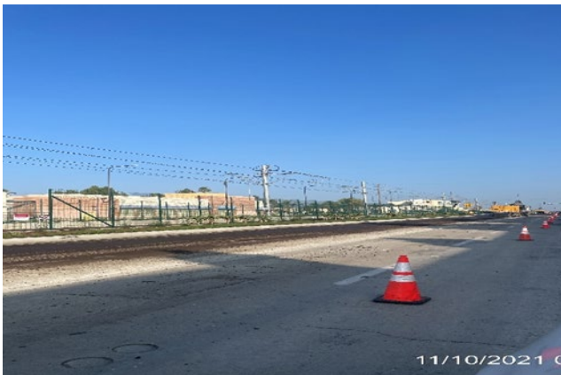
PARK MESA STATION – Continue street restoration northbound Crenshaw Blvd between 57th St and 54th St.
