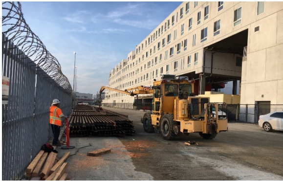
Rail Strings at the Division 20 Yard
