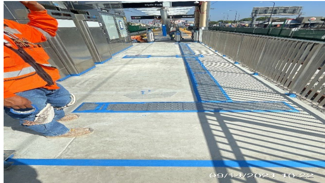
HYDE PARK STATION – Preparing the floor surface at the south end entrance ramp for coat finish placement.
