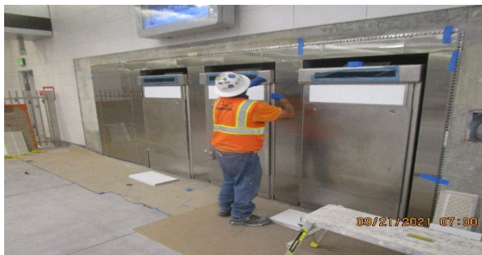
MLK STATION – Continue stainless steel cladding installation to the ticket vending machines at Free Area.
