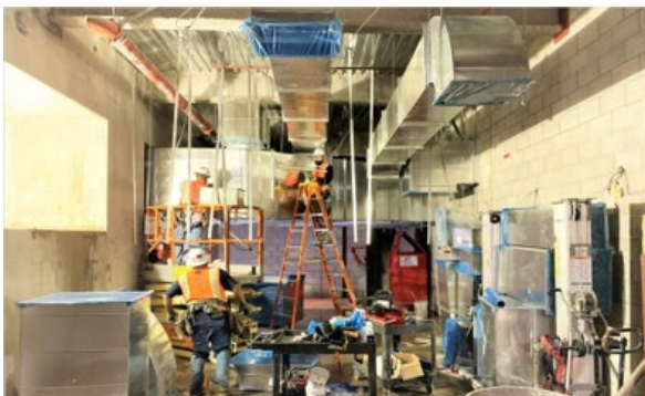
HVAC Installation at Wilshire/La Brea Station
