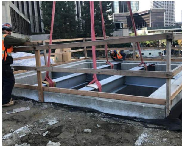
Welding support beams for supply air shaft at Grand Av Arts/Bunker Hill Station
