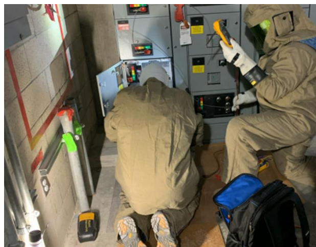
Testing voltage and phase rotation at Grand Av/Arts District Station
