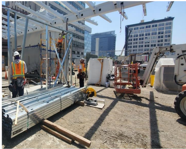
Installation of steel stud framing for plaza electrical closets at Historic Broadway Station
