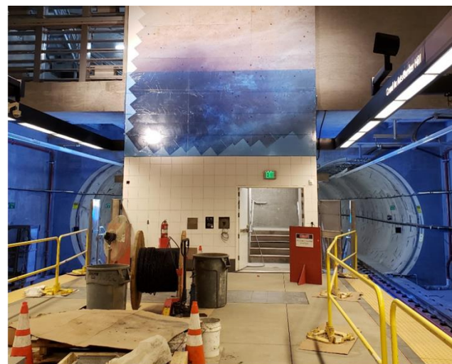
Hope PES Art – platform end wall at Grand Av Arts/Bunker Hill Station
