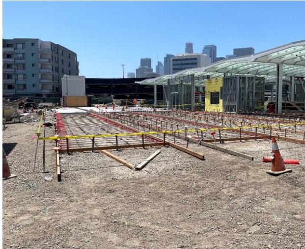
Plaza form and rebar for architectural paving at Little Tokyo/Arts District Station
