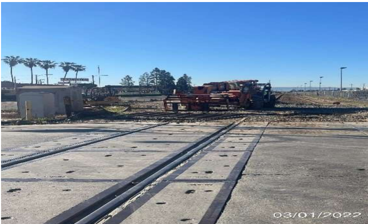
PARK MESA – Continue excavating soil in preparation for asphalt placement at the 67th Yard.
