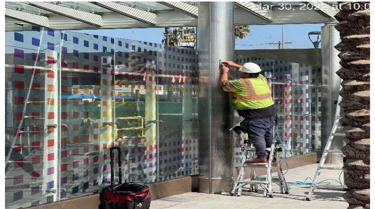
EXPO STATION – Applying anti-graffiti shield to the main entrance canopy columns at the plaza.
