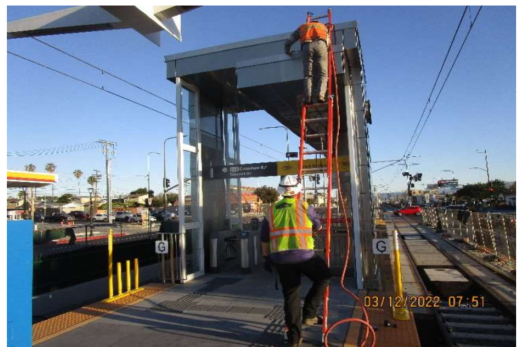
HYDE PARK STATION – Performing water pressure testing for the roof drains at the south pavilion.
