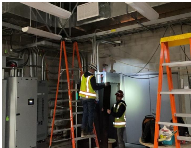
Installation of comm rack power receptables at Grand Av Arts/Bunker Hill Station TC&C Room
