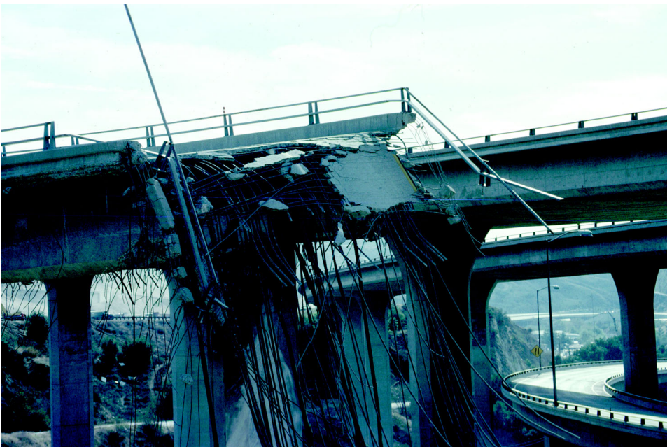
Figure 1. Northridge Earthquake Freeway Destruction
