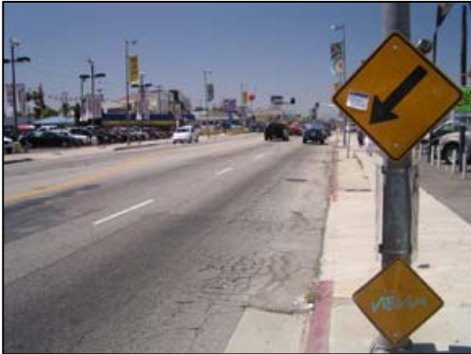
Rough pavement on Lankershim Blvd., looking north from Killion Street
