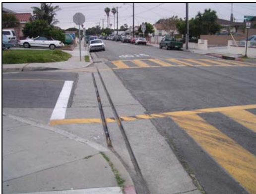
Slots in the valley gutters at Grevillea Ave and 166 th St
