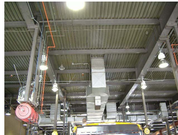
Divisions 3, 8, 15, and RRC Shop Lighting
