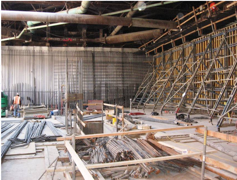
1 st /Boyle Mariachi Plaza Station - Concrete for upper mezzanine level walls are underway. All lower level walls have been completed at the track level.
