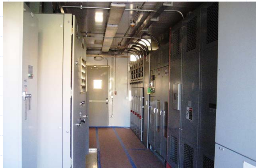
Traction Power Sub-Station 6 Interior
