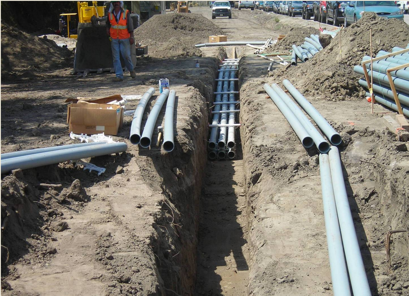
6-Way Ductbank in Segment B
