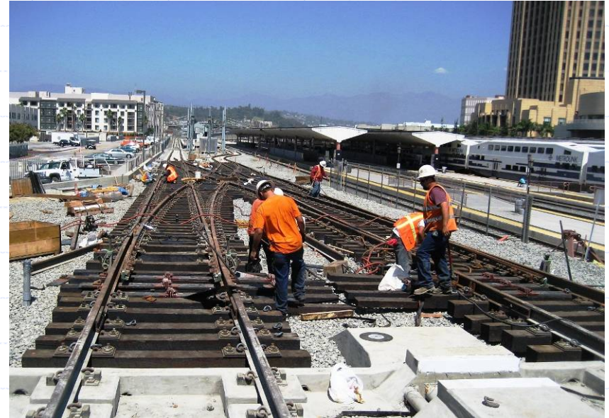
Track cross-overs were installed at Union Station to tie-in to the Pasadena Gold Line.
