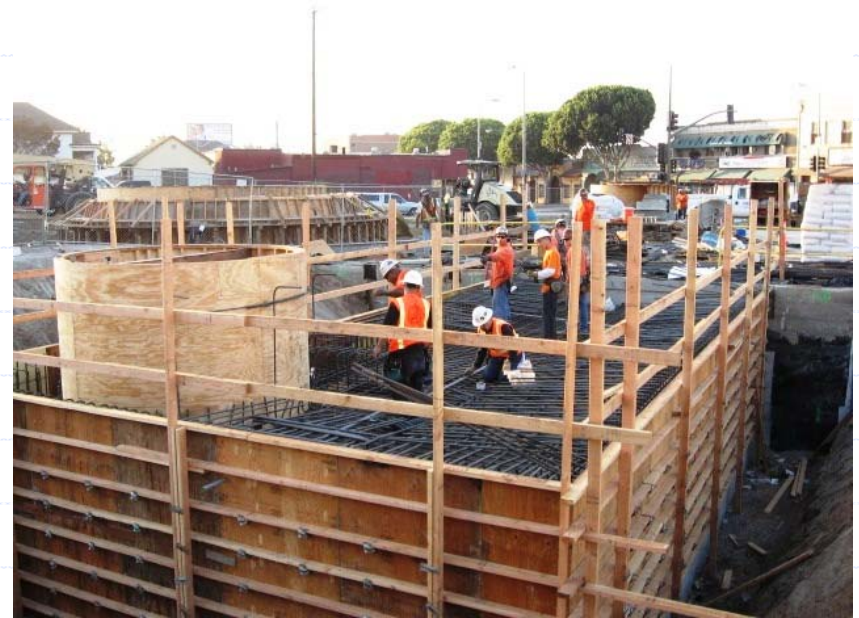
Soto Station - Southwest corner of 1st/Soto where the station entrance is being constructed in the future pedestrian plaza.
