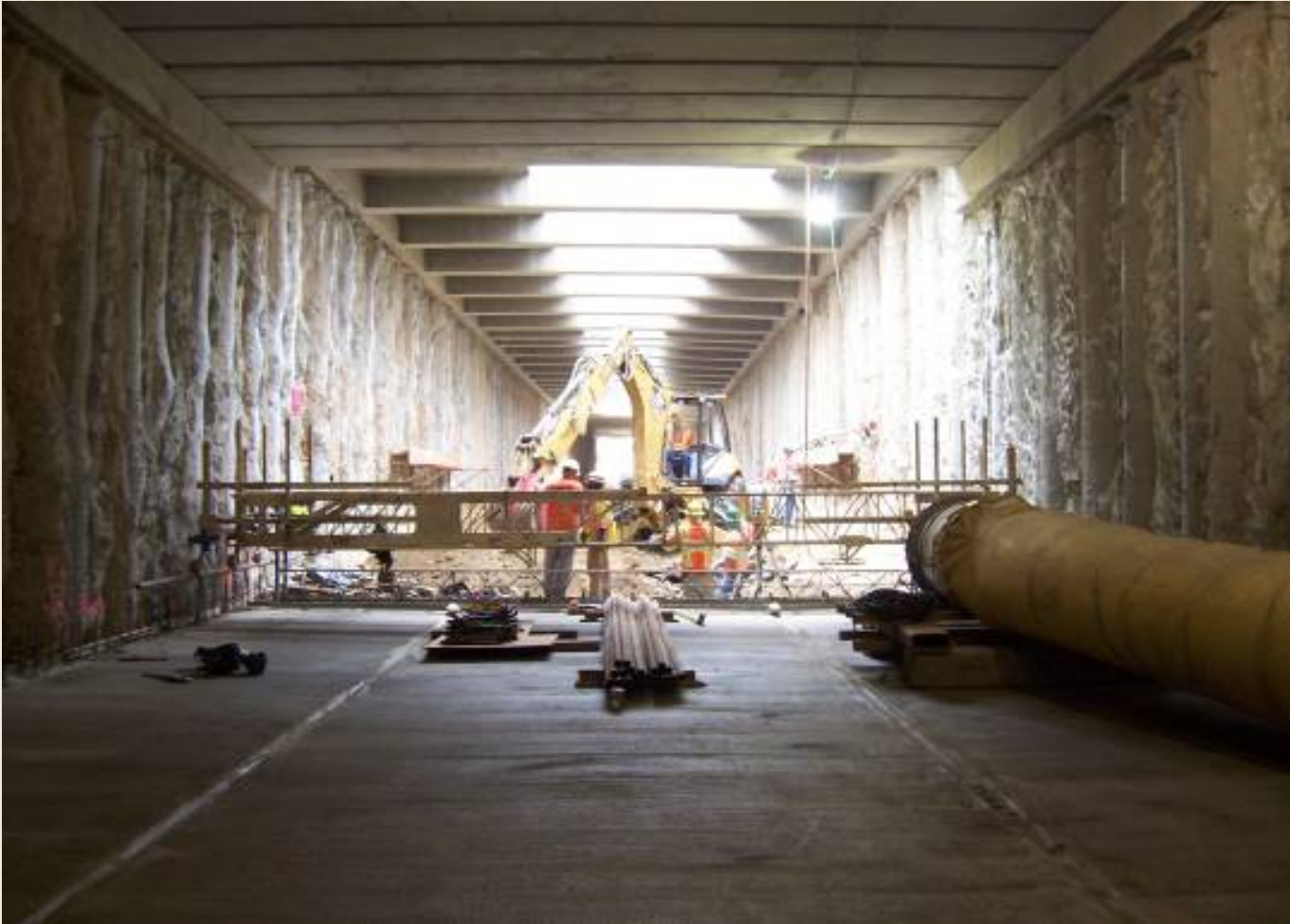
Sub-grade Preparation in Support of Invert Slab Placement at Grade Separation Trench Structure
