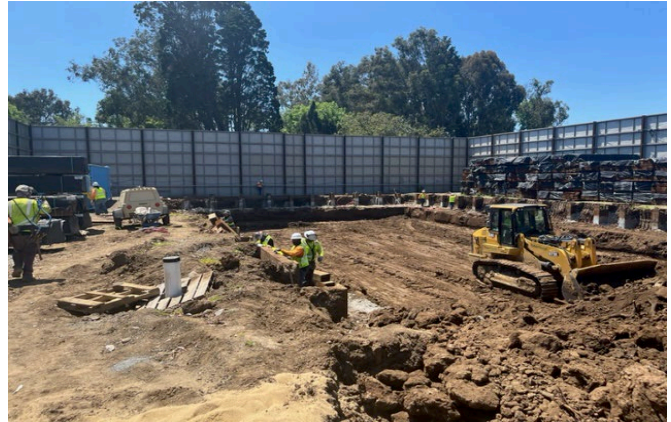
Westwood/VA Station: Installation of Level 1 Lagging and Waler Supports (at Bonsall Facing West)
