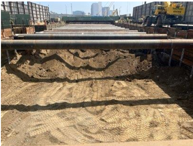
Westwood/VA Station: Installation of Level 1 Struts Between GL22 & GL44, West of Bonsall
