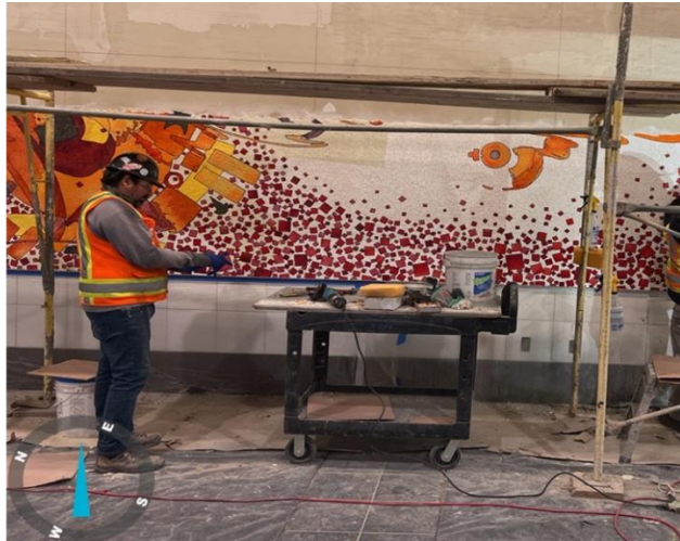
Mosaic art glass installation progress along north wall at Historic Broadway Station
