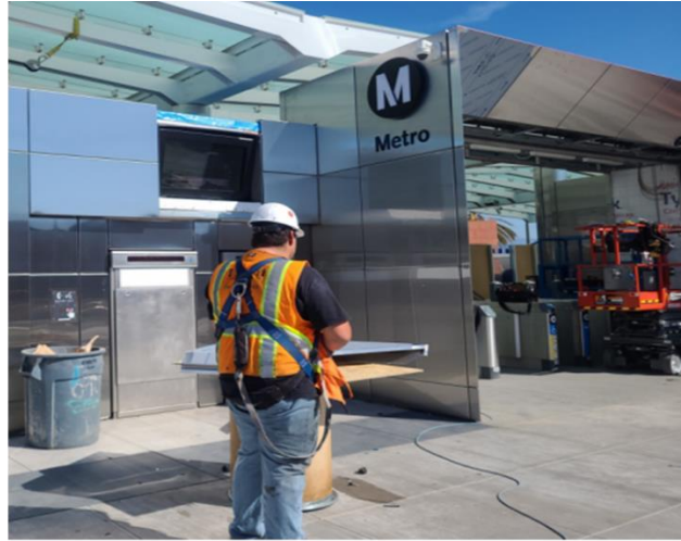
Stainless steel cladding installation at south entry portal at Little Tokyo/Arts District Station
