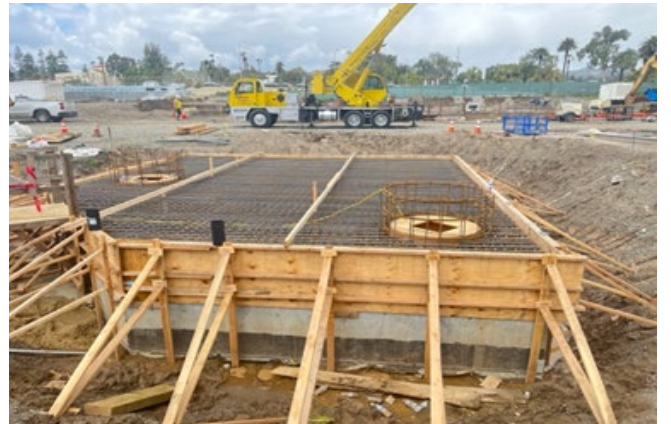
VA Steam Tunnel – Installation of Formwork, Shoring & Reinforcement for Vault 300 Roof Slab
