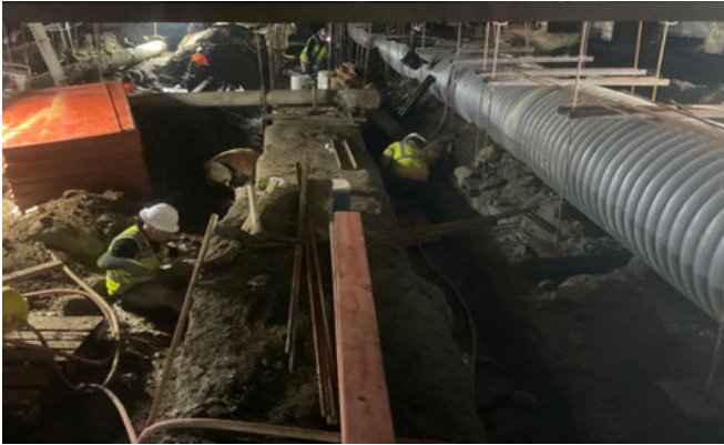
Westwood/UCLA Station: Installation of Level Two Lookouts on Southern Wall of Station Box
