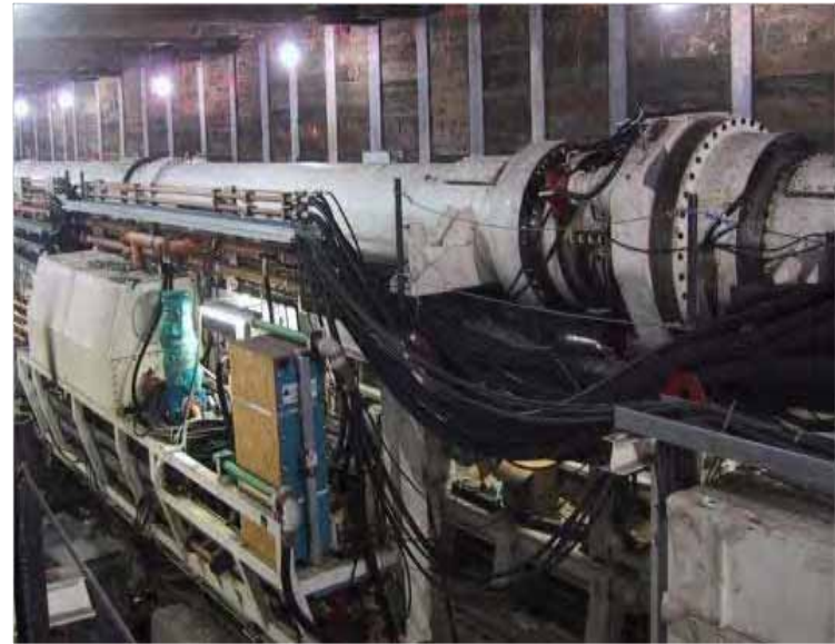
Figure 5-6: EPBM Screw Conveyor for MGLEE
