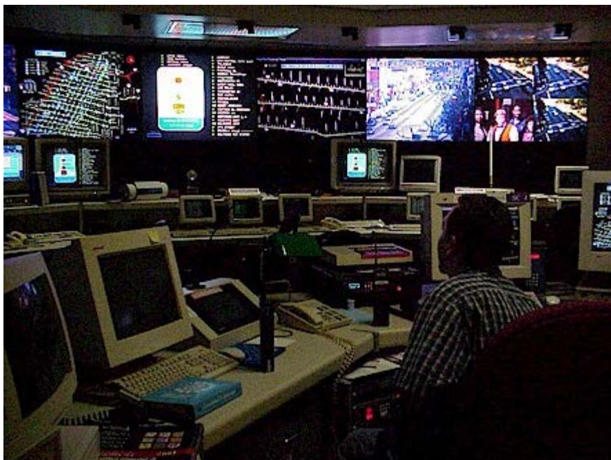
The ATSAC center beneath City Hall East reminds a visitor of the MTA's Rail Operations Control center at Imperial/Wilmington.
