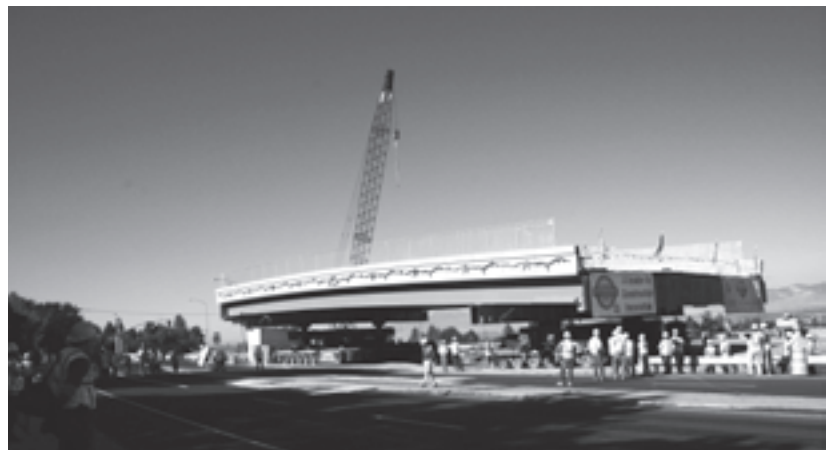
Bridge construction in Utah deploys self-propelled modular transporters, an innovative technique examined in SHRP 2 renewal research. (Photo: Utah Department of Transportation)
