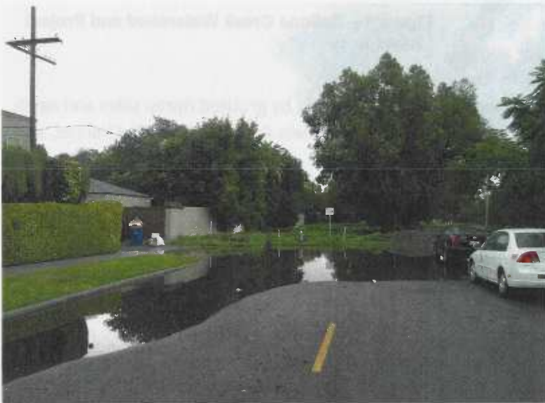
Figure 3 – Water Ponding at Exposition Blvd and Westwood Blvd (North Side)
