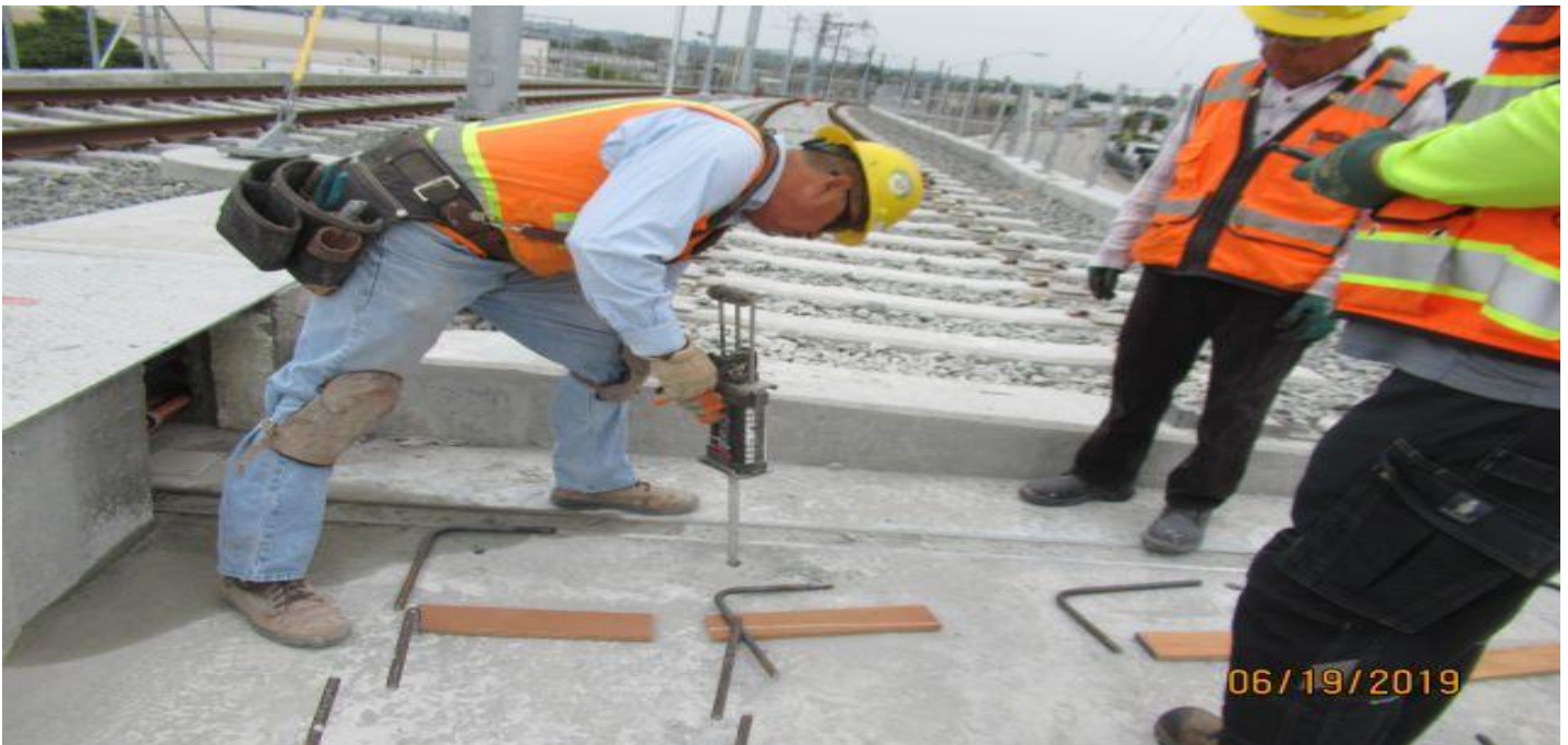
MANCHESTER BRIDGE- WSCC applying epoxy into hole for installing rebar onto deck plate.
