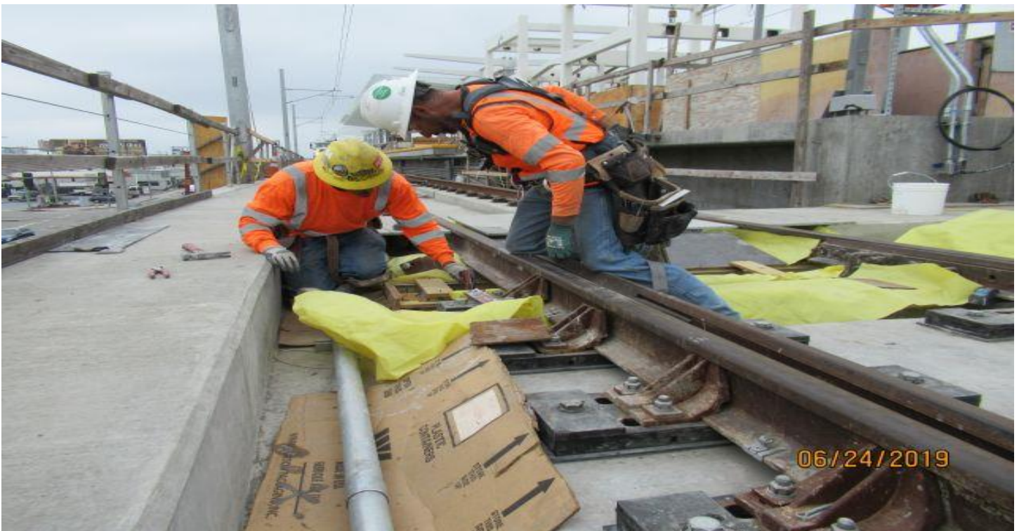
AVIATION/CENTURY- WSCC repairing concrete forms prior to placing concrete on K1LH XO Century bridge.
