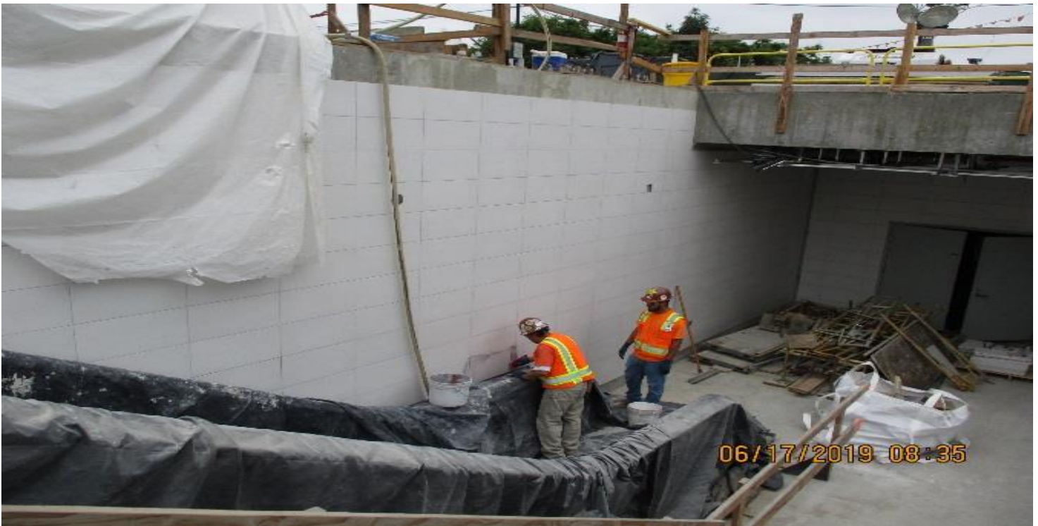
LEIMERT PARK STATION- Continued tile grout from mid landing to plaza at entrance stairs #1.
