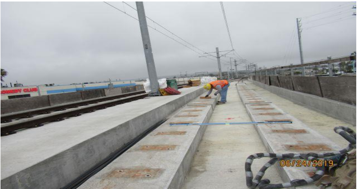
MANCHESTER BRIDGE- WSCC finisher verifying fastener plane on L&R plinths Manchester bridge.
