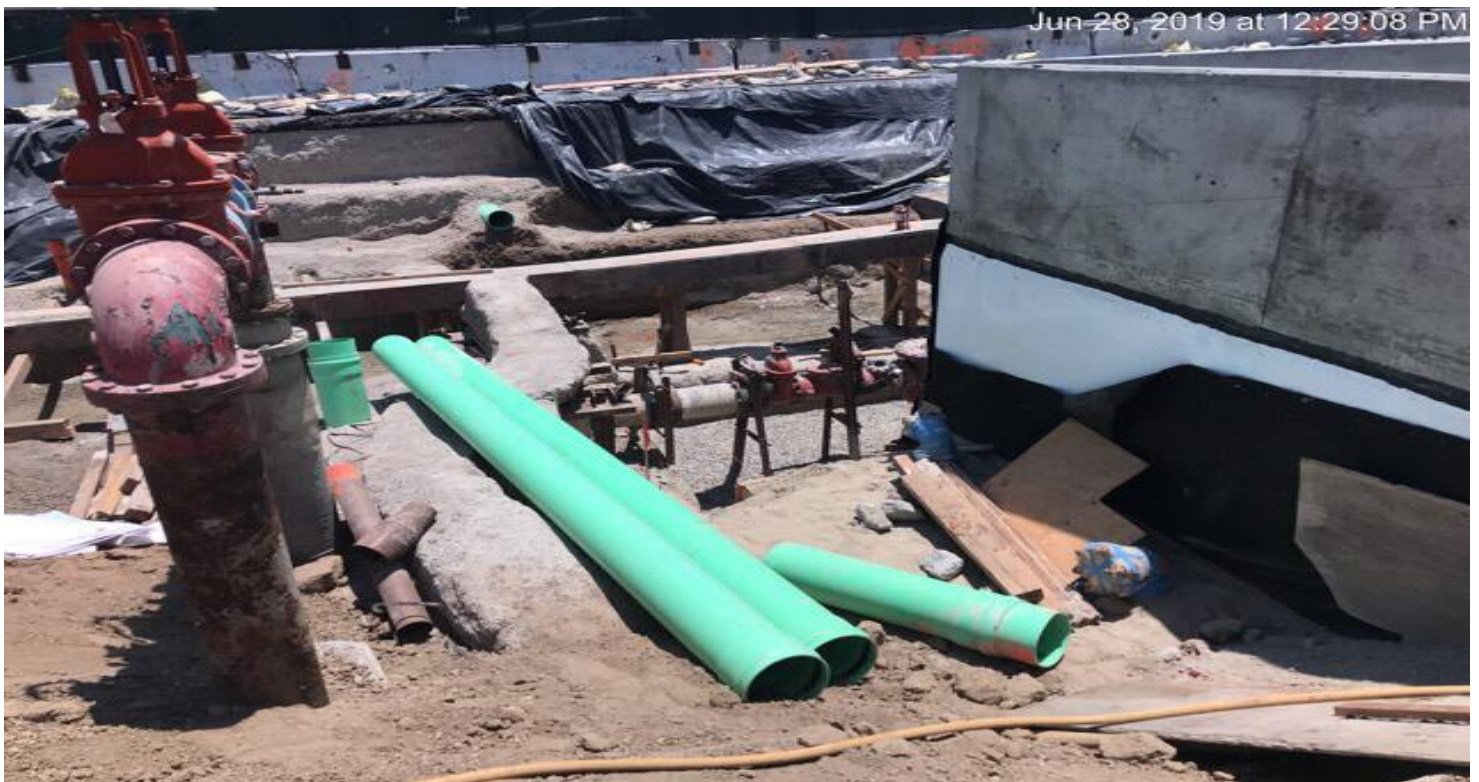
MARTIN LUTHER KING JR. STATION- Layout form for water line vault at the topside.
