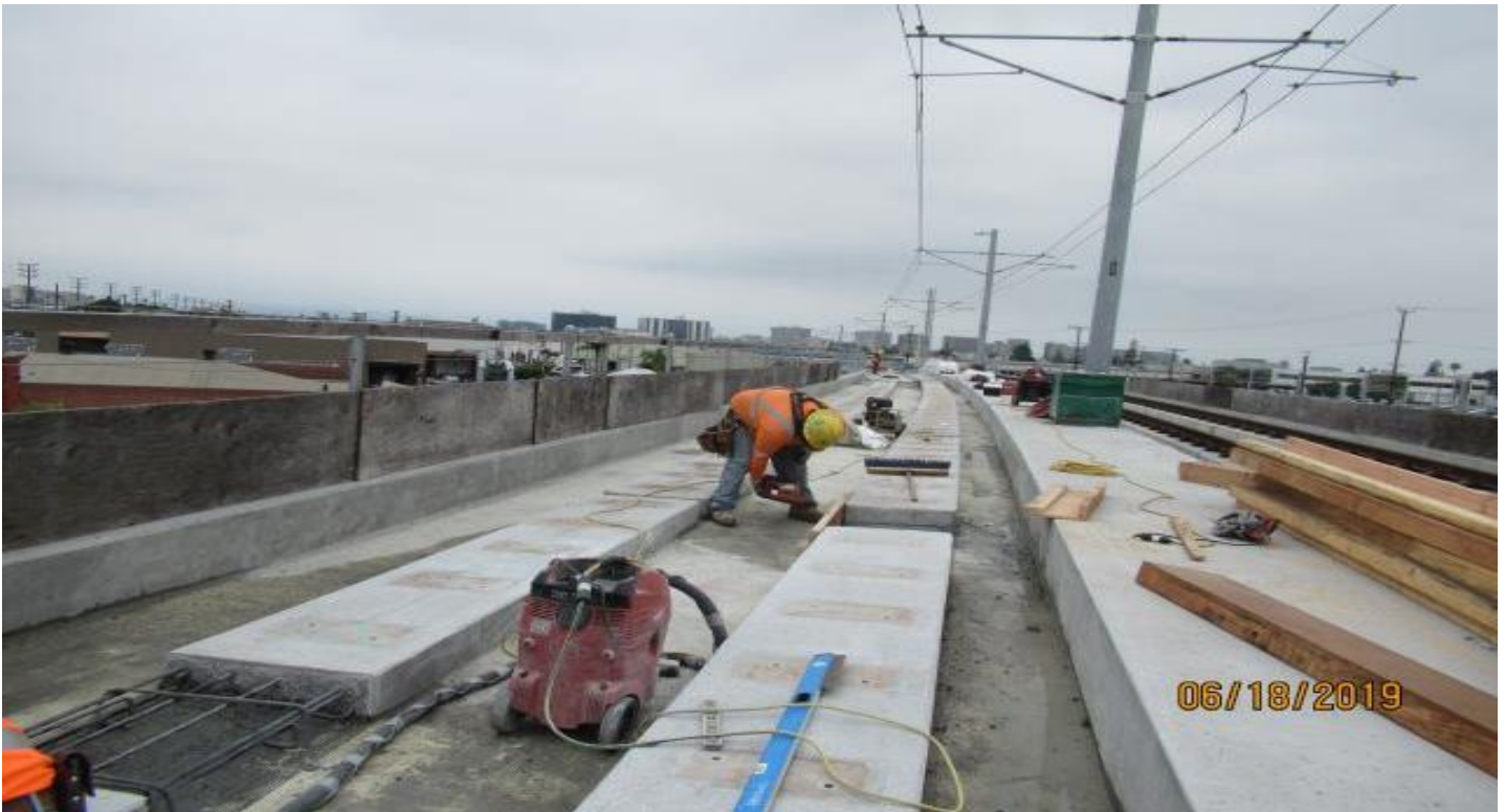
MANCHESTER BRIDGE- WSCC framing up forms for placing concrete into plinth NB track Manchester Bridge.
