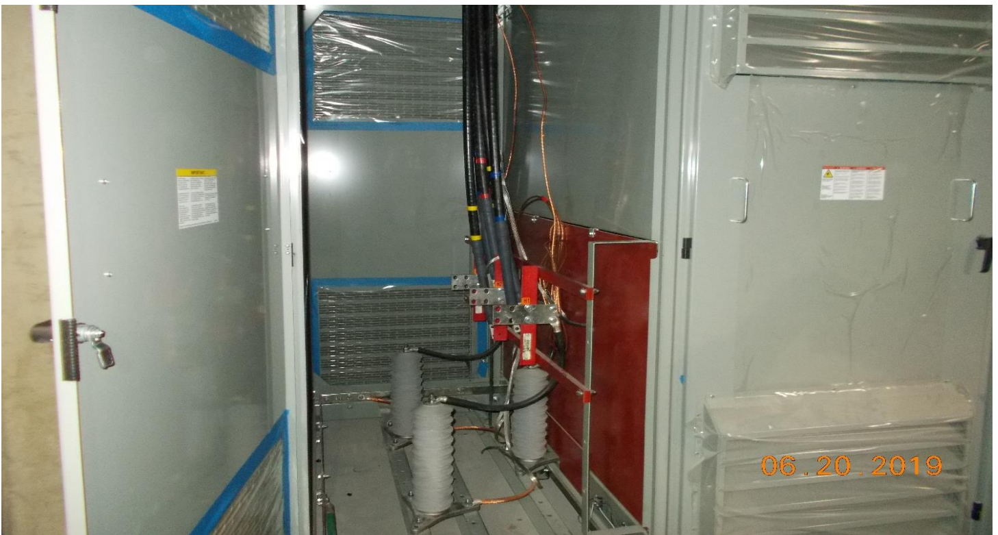
CRENSHAW/VERNON- PX1S high voltage terminations on cables.
