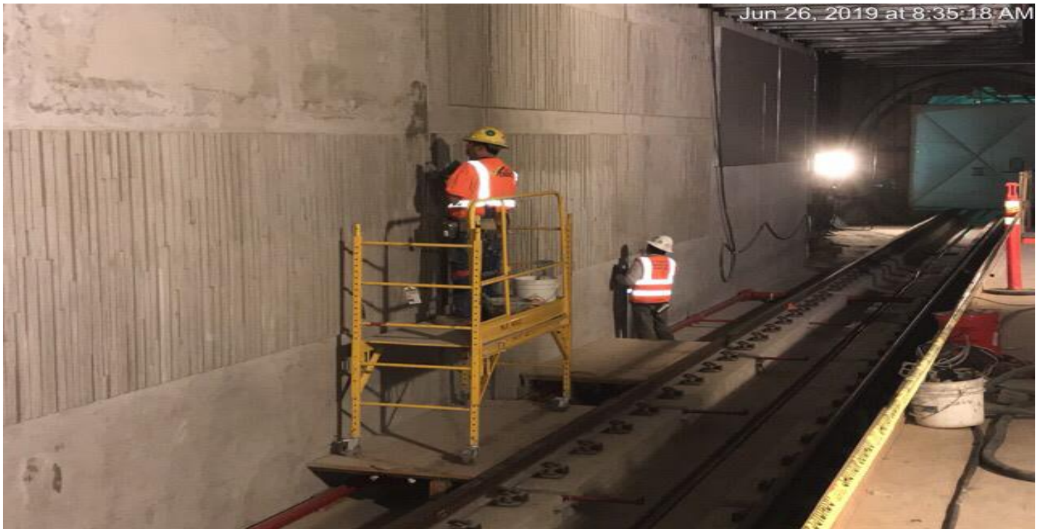
MARTIN LUTHER KING JR. STATION- Continued finish work from invert to concourse level at Emergency Exit #2.
