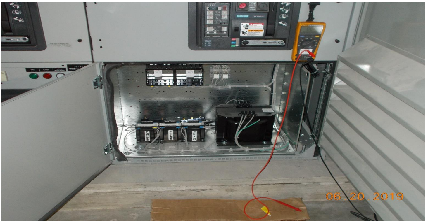
CRENSHAW/EXPO- Aux Power room south, NETE installing shunts and disconnecting electronics for electrical testing on MSWGR.
