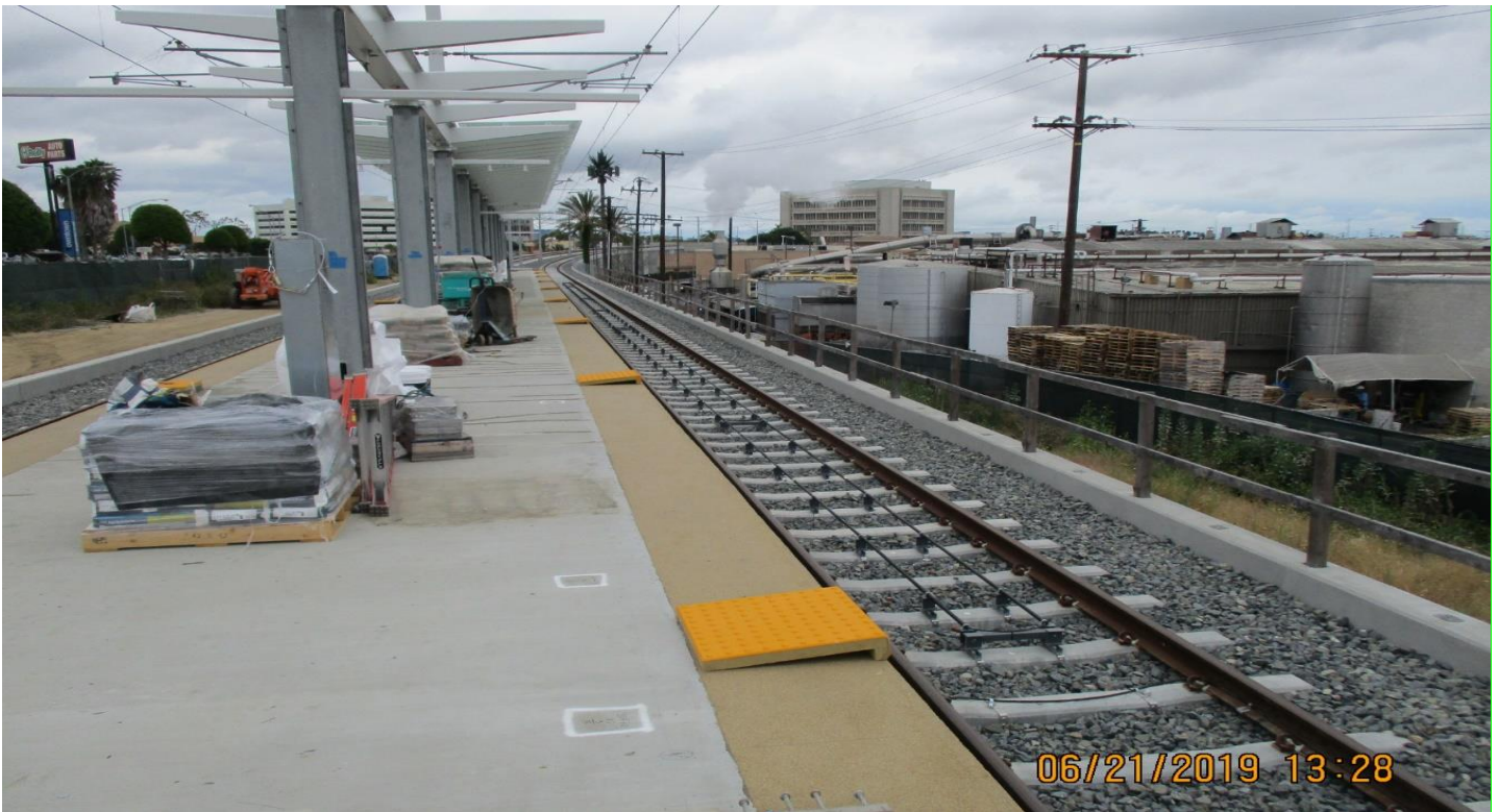
DOWNTOWN INGLEWOOD STATION- Guideway at Downtown Inglewood Station platform and ticketing pavilion overview.
