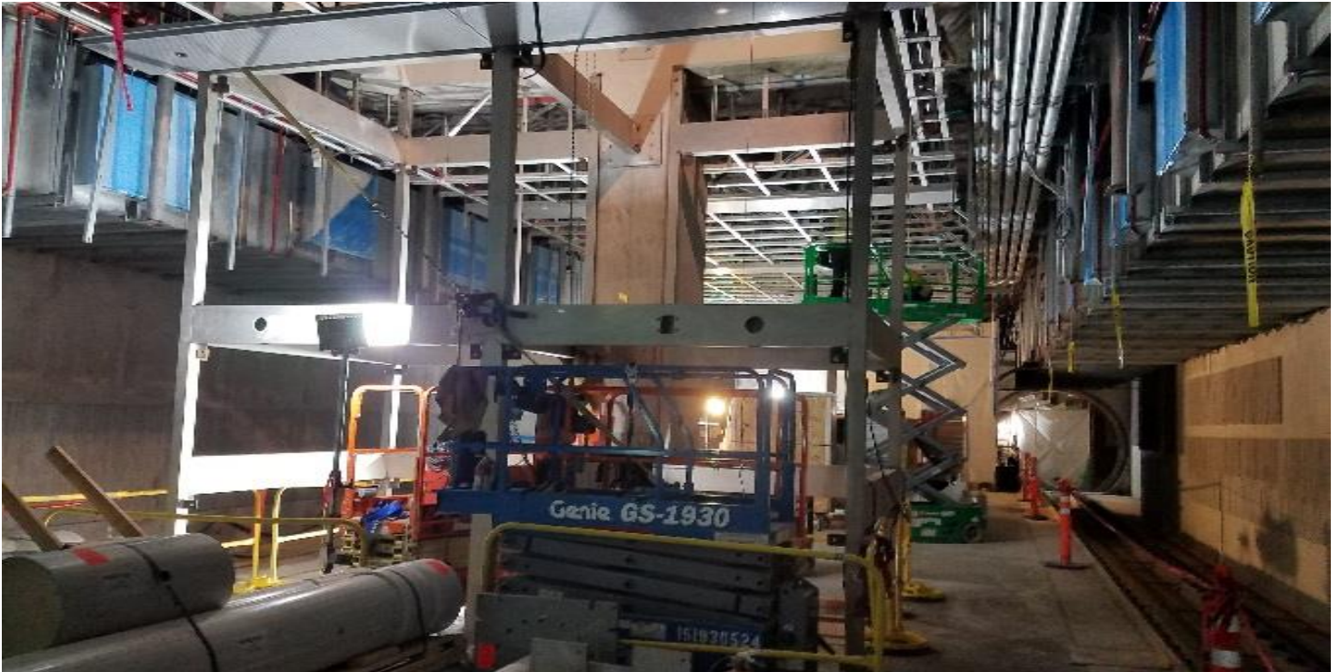
LEIMERT PARK STATION- Continued installation of elevator frame 3 & 4 at the platform level.
