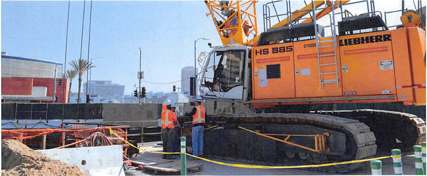
Construction equipment powered by renewable diesel in use at the Metro Regional Connector project
