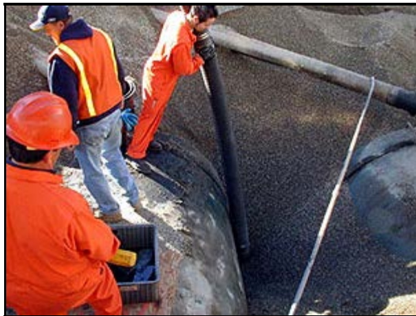
^ A crew excavates contaminated soil around a waste oil and chemical storage tank.
