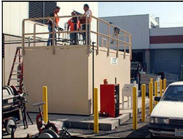
^ Workmen put the final touches on an aboveground diesel fuel storage tank at the RRC.
