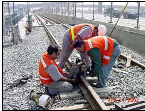
▲ Construction crew members work to modify the Metro Green Line tracks at the Harbor Freeway station.
