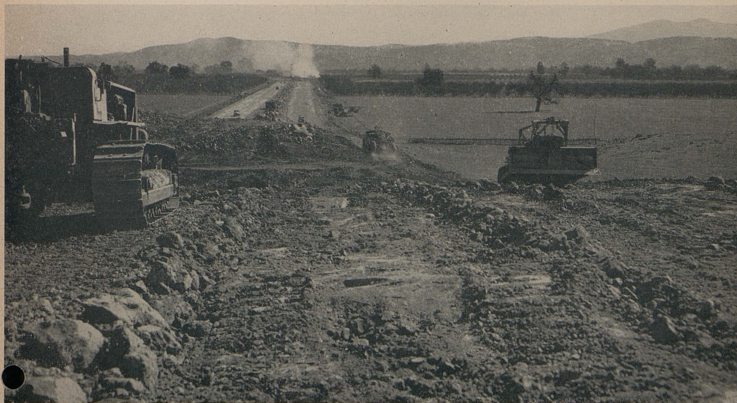
Rock cut being excavated and hauled to fill. Smoke in background is from burning brush in clearing operations.
