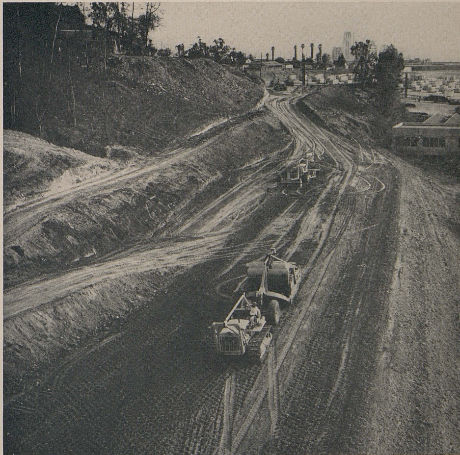
Looking south from existing Sixth Street Bridge, showing a fill in process of construction
