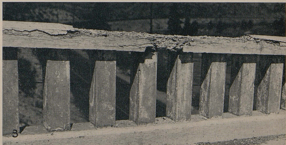
This photo shows concrete deterioration on Polaris Bridge
