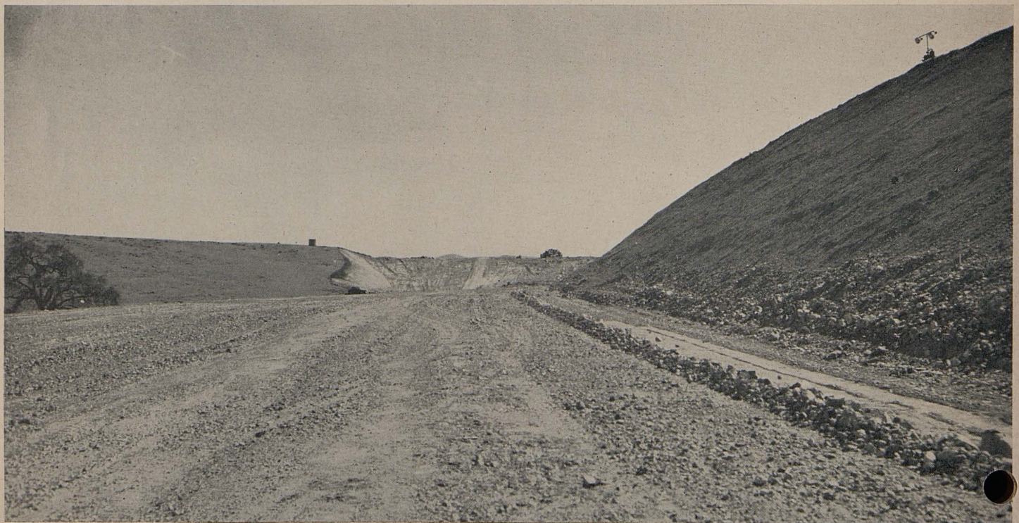
This photograph, looking south, shows completed rough grade in side hill cut
