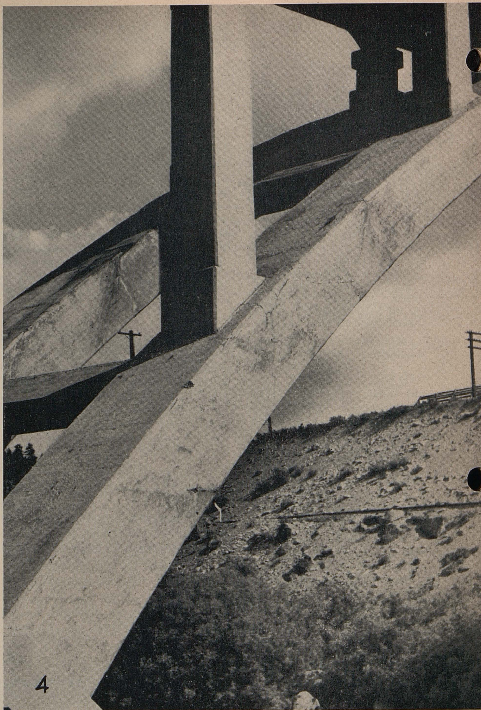
Portions of arch ribs of Polaris Bridge have disintegrated
