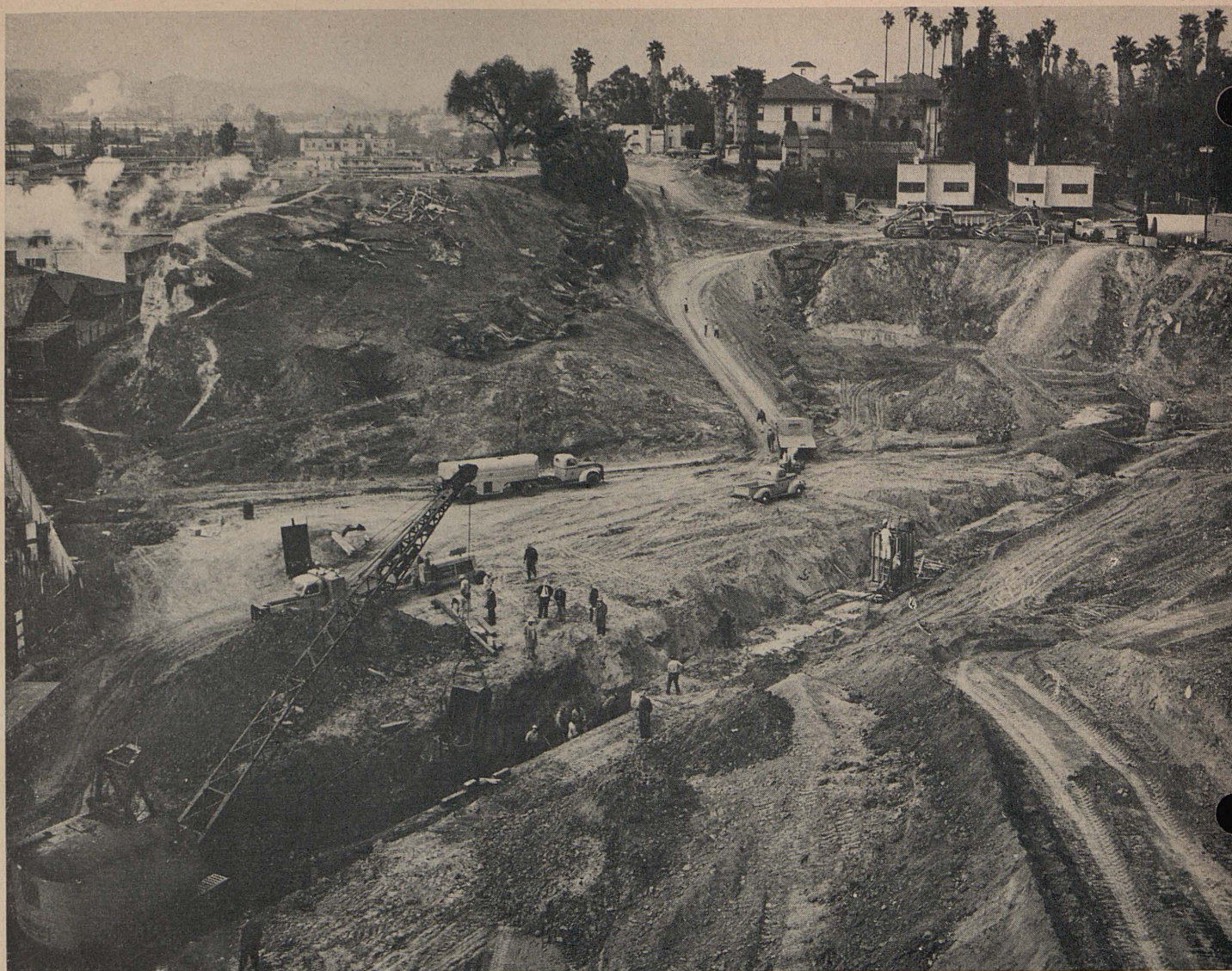
Looking northerly from Sixth Street Bridge. In foreground reinforcing of an existing storm drain which will be under quite a high fill is in progress
