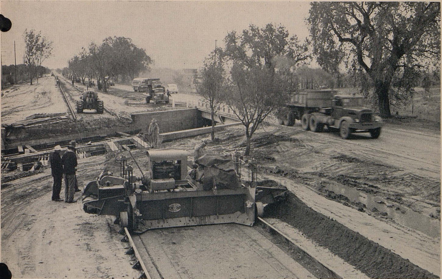
Showing position of new lane in relation to the existing lane. Material between steel headers is cement treated base with curing seal applied
