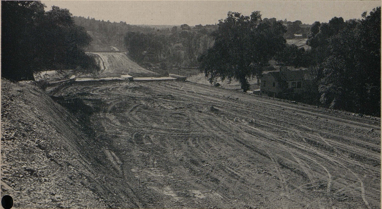
Upper—Grading equipment constructing fill near Southern Pacific Overhead. Lower—Looking west across Walsh Street Undercrossing during construction
