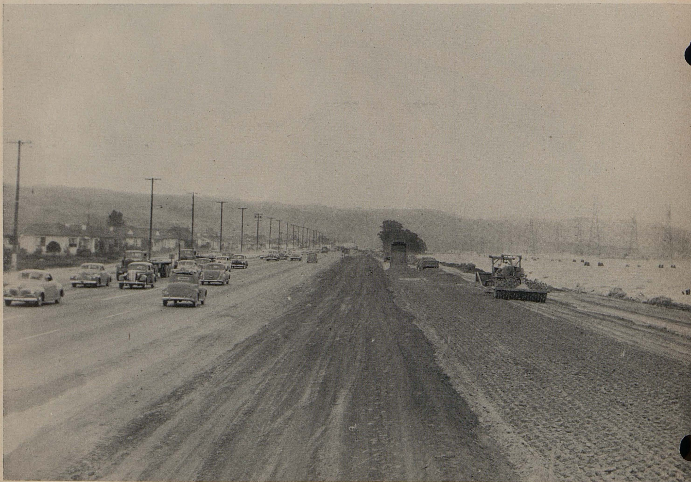
Looking north on Bayshore project, showing construction of fill for northbound freeway section. Traffic is on present traveled way
