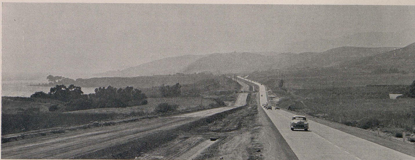
This expressway under construction south of Santa Barbara is another link in the chain of improved sections on US 101. In this photo, the new lanes have been completed and are being used by traffic while the old roadway to the left is being reconstructed to expressway standards.
