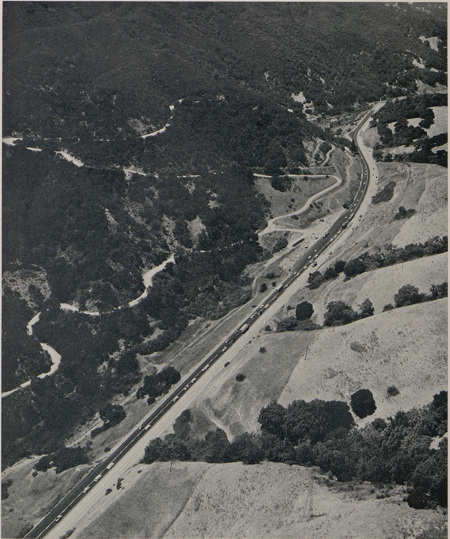
Traffic was routed along the completed two-lane section during reconstruction of US 101 on the Cuesta Grade in San Luis Obispo County. The winding road on the slopes to the left is the pre-1937 highway.
