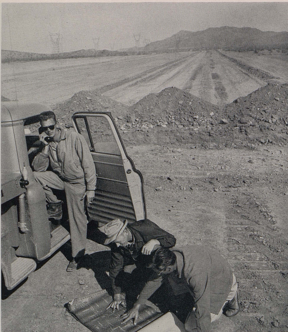
Inspectors using radio to check blueprints out in the wide open spaces on the Victorville-Barstow expressway are, left to right, W. T. Murray, Art Austin and R. H. T. Norton
