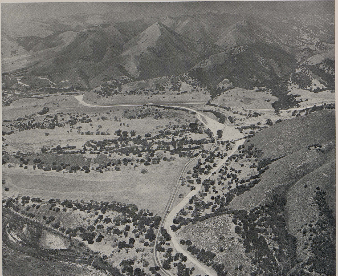
Clearing and grading for the relocation of Sign Route 166 along the Cuyama River can be seen as a lighter line following the general location of the present highway in this aerial photo
