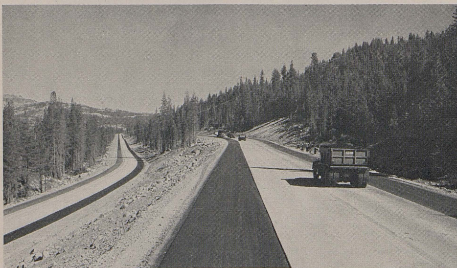
Hampshire Rocks to Soda Springs portion just before completion while crews were completing asphalt shoulders.
