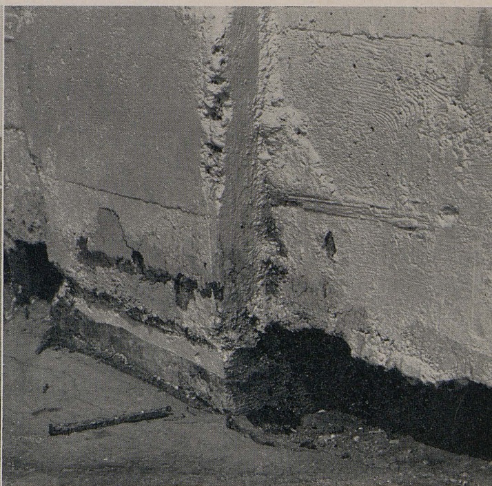
Floor actually sank beneath foundation footings in places. Pile cap is almost exposed at this point.
