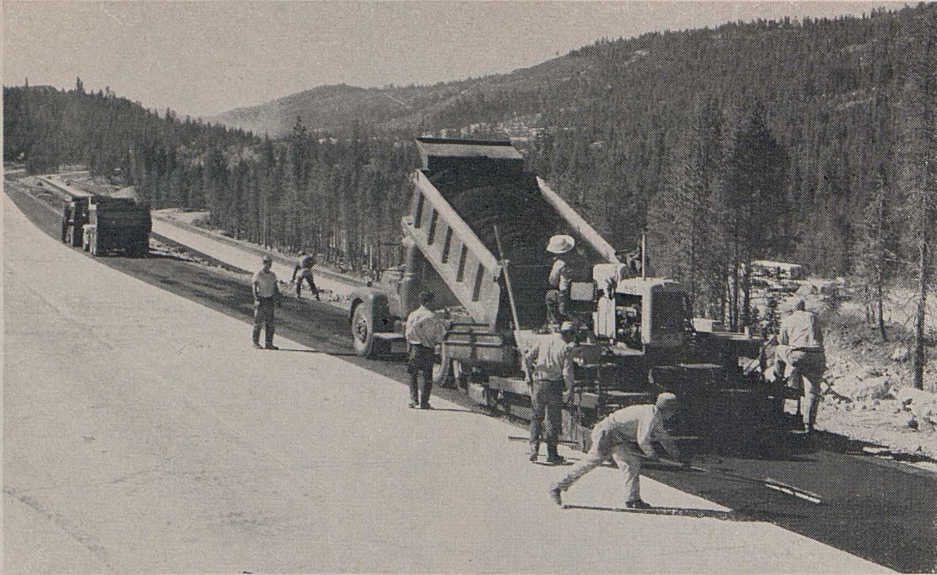
Contractor's crews finishing asphalt shoulder on Hampshire Rocks to Soda Springs section.
