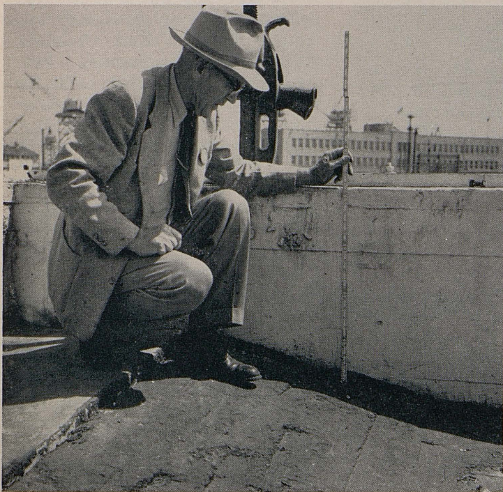
Slab floor of old building settled seriously on tide land fill. Archie Prescott of Navy Public Works here shows where supplementary asphalt ramp had to be built to accommodate warehouse rolling stock.
