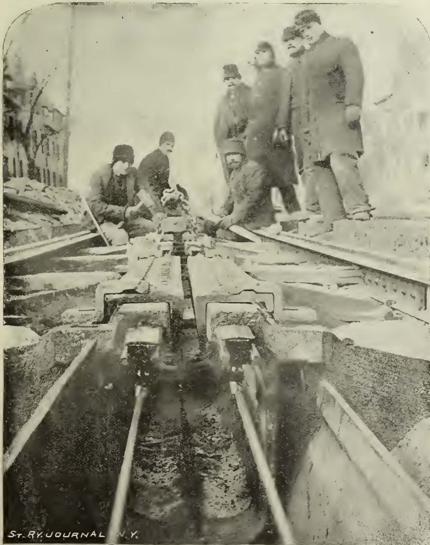
FIG. 2.—STREET SCENE—CHICAGO UNDERGROUND ELECTRIC SYSTEM.
