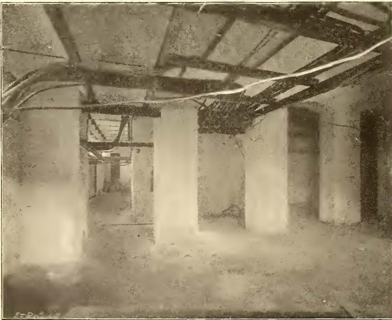
FIG. 8.—VIEW OF FEEDER VAULTS—13TH STREET STATION OF PHILADELPHIA TRACTION CO.
