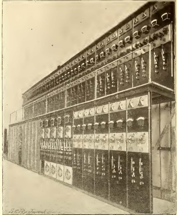
FIG. 5.—SWITCHBOARD—13TH STREET POWER STATION OF PHILADELPHIA TRACTION CO.
