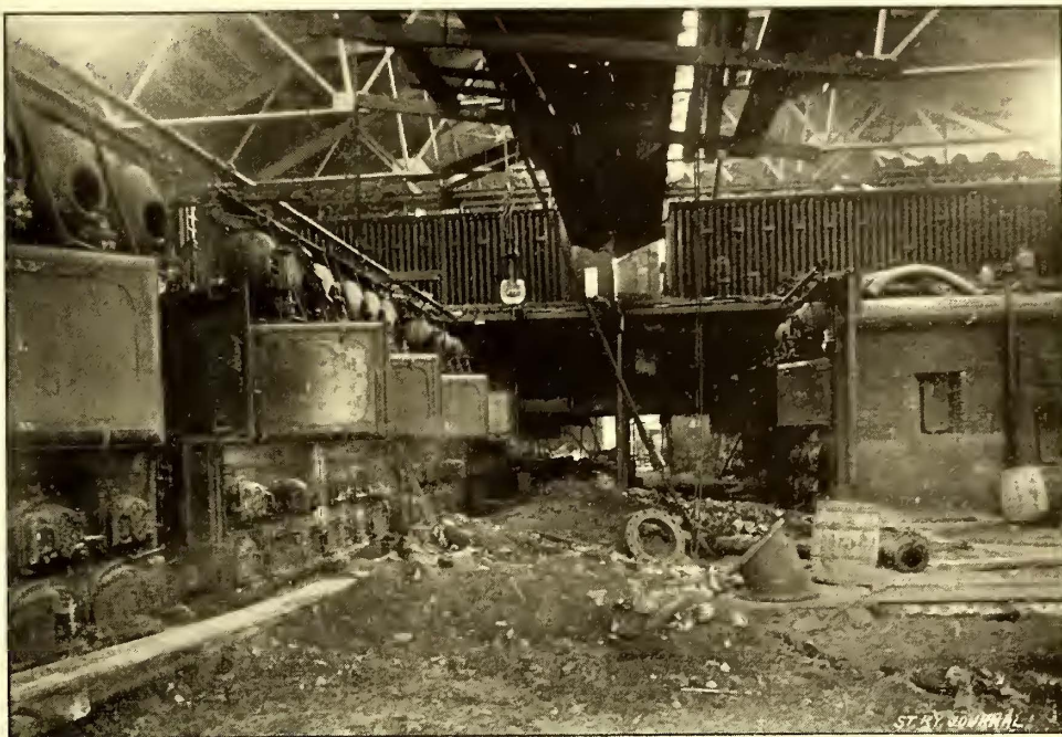
FIG. 8.—VIEW OF BOILER ROOM, DELAWARE AVENUE POWER STATION—ELECTRIC TRACTION CO., PHILADELPHIA.
