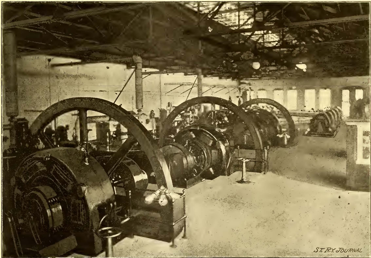
FIG. 1.—INTERIOR OF POWER STATION—JERSEY CITY.
