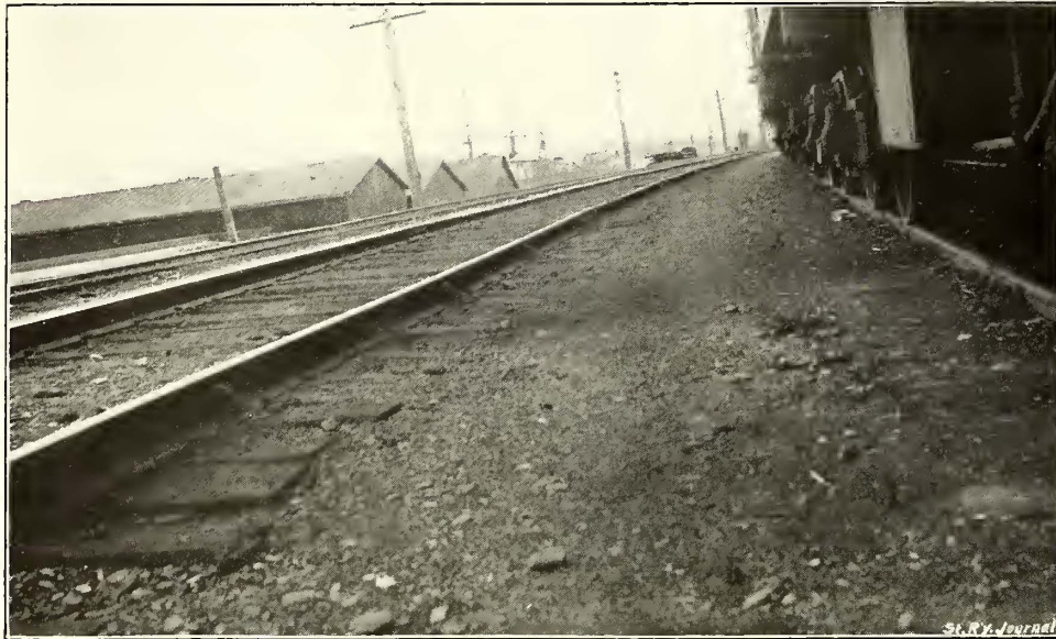
FIG. 5.—AN ILLUSTRATION OF RAILROAD TRACK LAID WITH POOR JOINTS.
