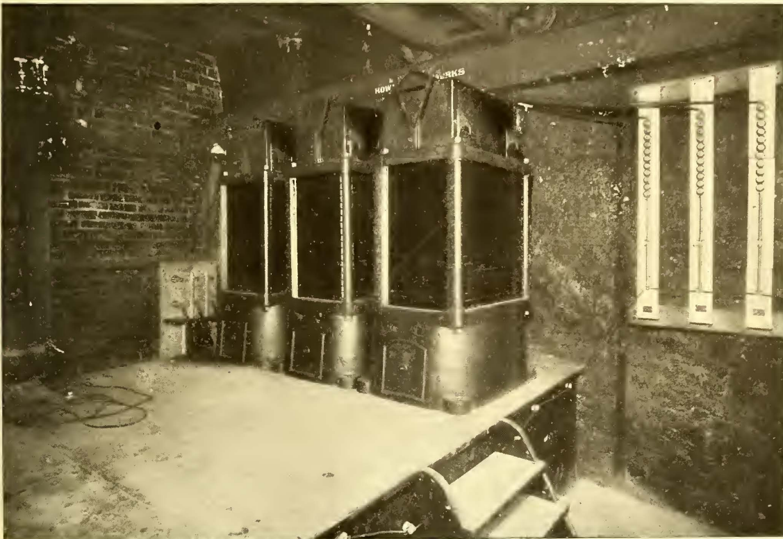
FIG. 2.—INTERIOR OF STEP-DOWN TRANSFORMER STATION—BUFFALO.
