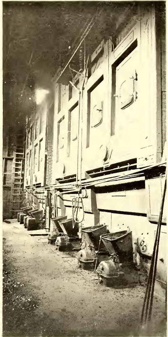
BOILER ROOM, AKRON
