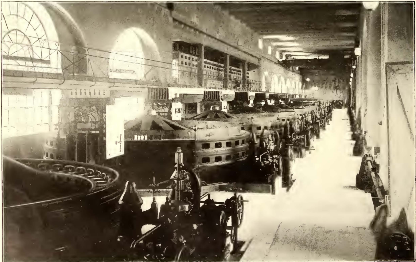
CHEVRES POWER STATION, GENEVA
