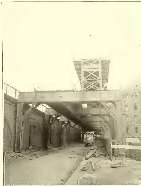
FIG. 15.—GENERAL VIEW OF ELEVATED STRUCTURE, WITH TEMPORARY TRACK FOR TRANSPORTING MATERIAL ABOVE
