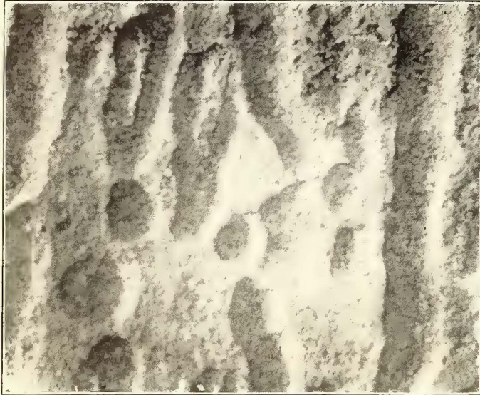
FIG. 5.—REPRODUCTION OF PITTINGS FROM STAND-PIPE IN RARITAN NOT DUE TO ELECTRIC RAILWAY
