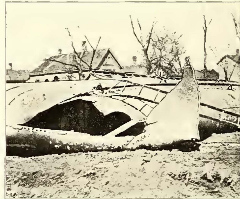
FIG. 1.—VIEW OF WRECKED STANDPIPE AT PEORIA, ILL., SHOWING PITTING ON UPTURNED PIECE, DUE TO ELECTROLYSIS
