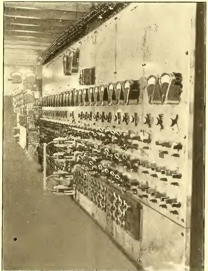
SWITCHBOARD IN CHARGING STATION
