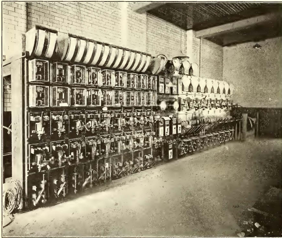
MAIN TRACTION SWITCHBOARD AT SALFORD STATION
