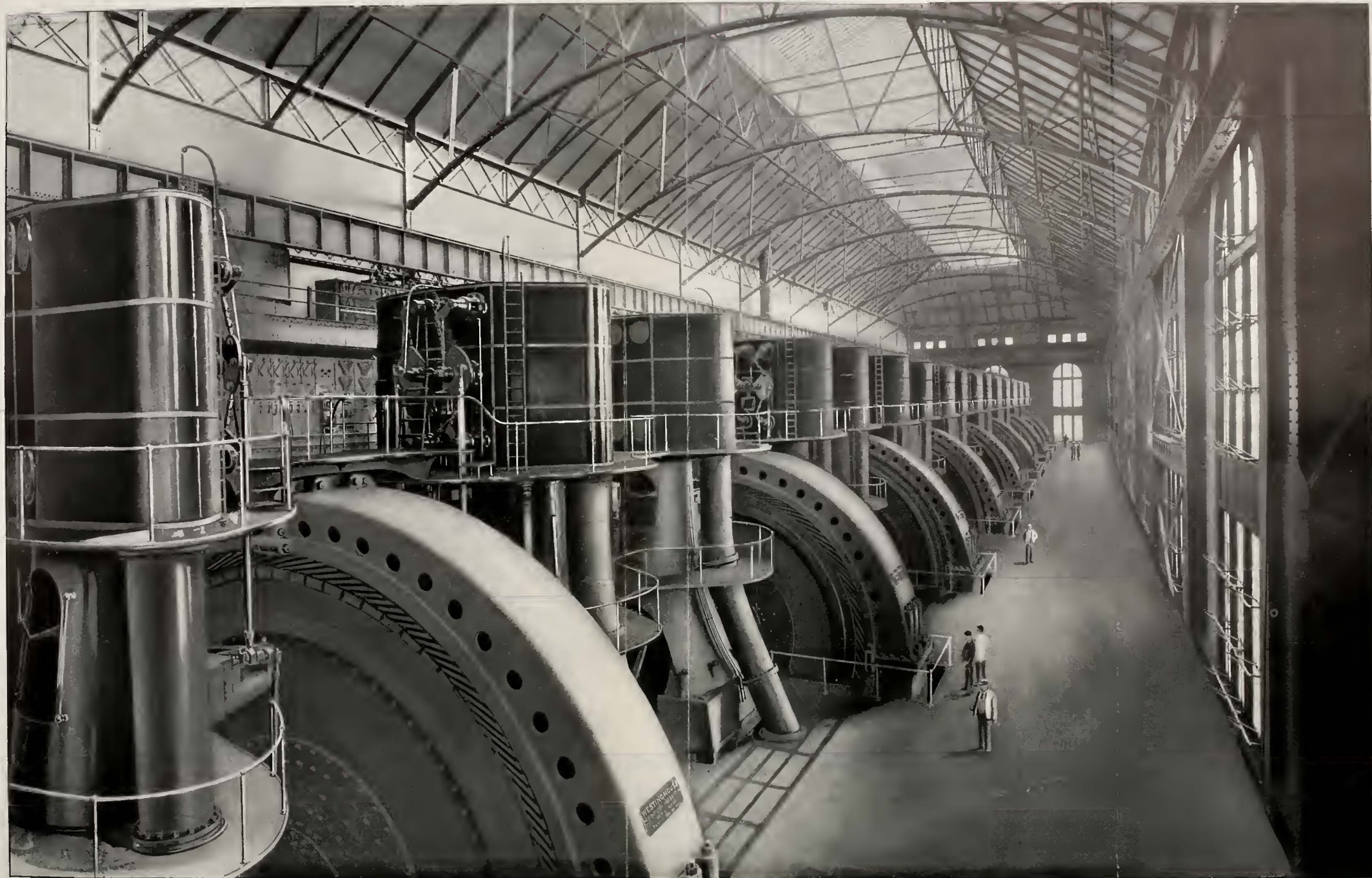
INTERIOR VIEW OF THE SEVENTY-FOURTH STREET STATION OF THE MANHATTAN RAILWAY CO. OF NEW YORK CITY, SHOWING EIGHT 8,000-H. P. GENERATING UNITS
