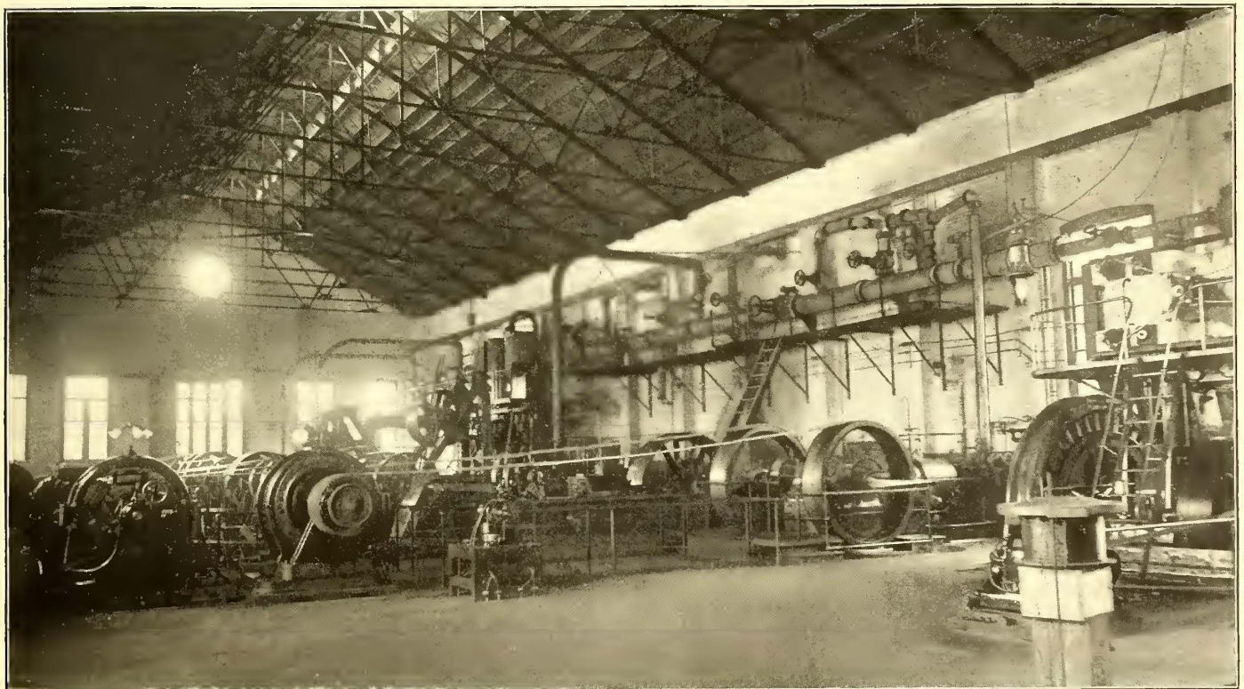
GENERAL VIEW OF ENGINE AND DYNAMOS
