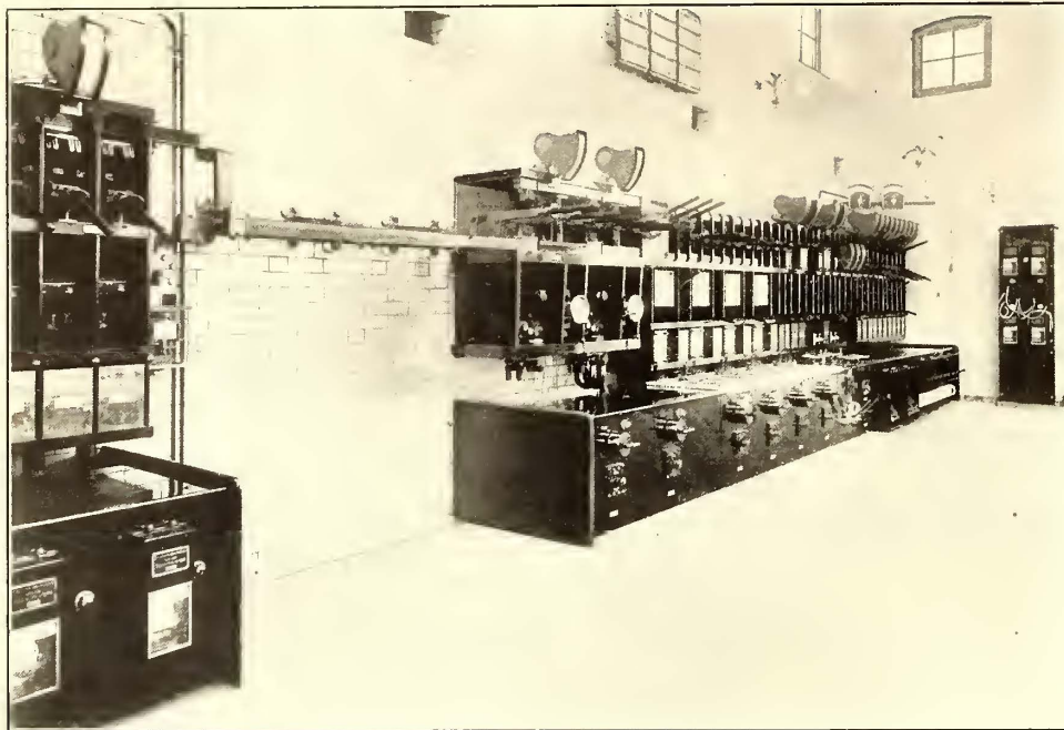
SWITCHBOARD FOR BOTH LIGHTING AND TRACTION CIRCUITS
