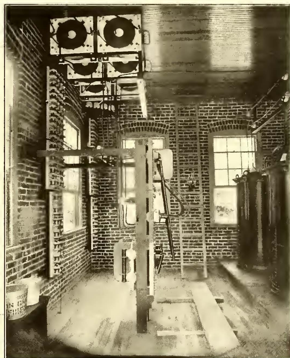
STATIC TRANSFORMERS IN SUB-STATIONS
