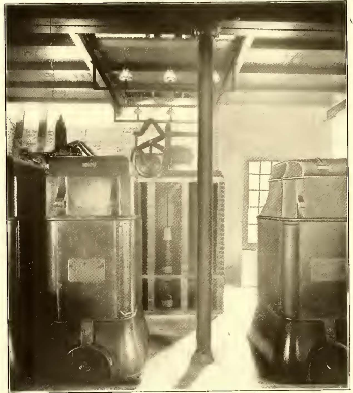
OIL SWITCH AND TRANSFORMERS IN SUB-STATION
