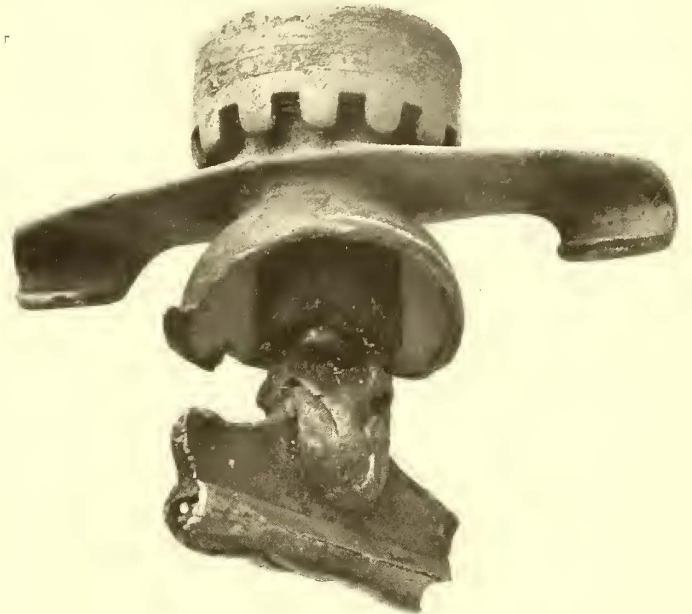
DAMAGED HANGER AND EAR
