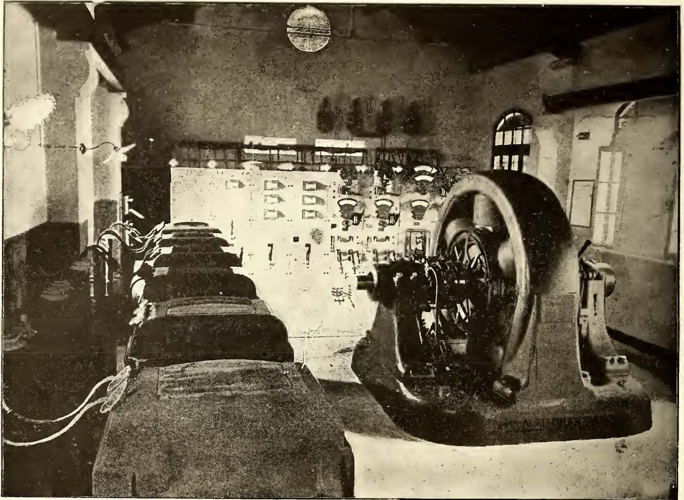
INTERIOR OF SUB-STATION AT PARABIAGO
