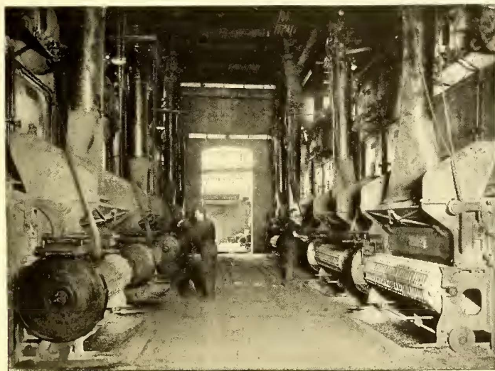
VIEW OF LOWER BOILER ROOM
